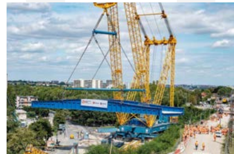
Works to replace the Chartres and Gallardon bridges, led by SNCF Réseau and RATP to improve efficiency on RER lines B and C.
