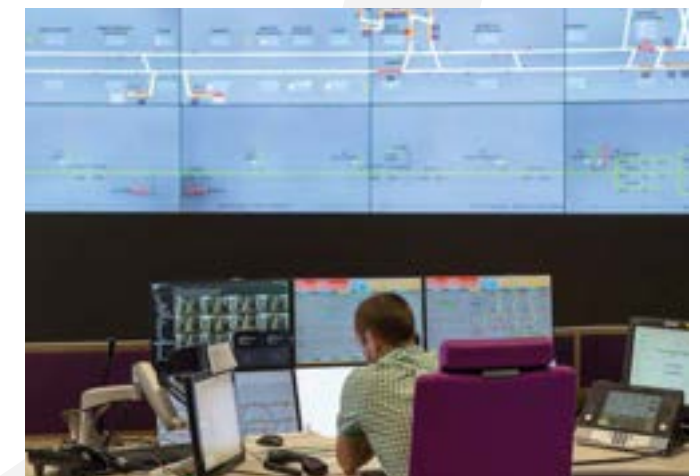
Metro line 4 central command post.
