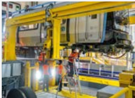
Metro line 11 train maintenance centre at Rosny-sous-Bois.
