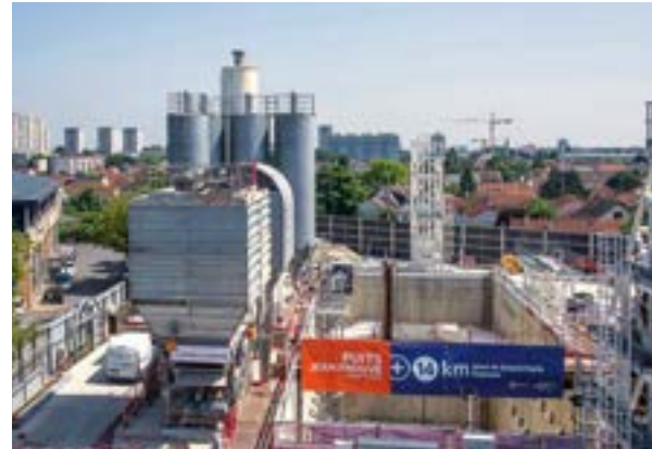
Tunnel boring machine (TBM) launching shaft in L'Hajj-les-Roses, metro line 14 southern extension work site.
